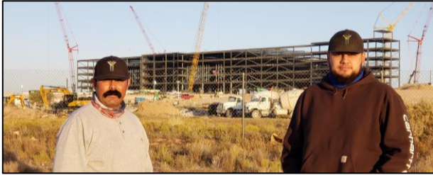
Max Varela , Foreman, & Martin Trujillo , 3 rd year apprentice. Amazon Fulfillment Center, Yearout Mechanical.
